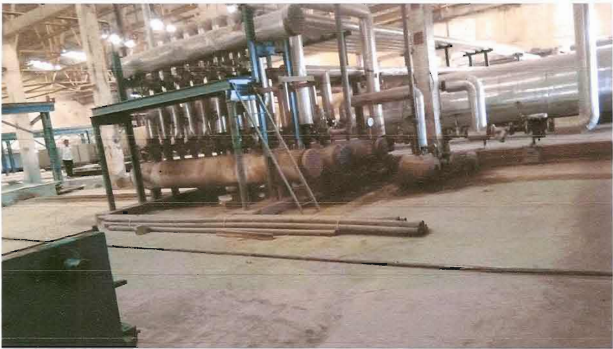
Plant & Machinery in Platinum AAC block
